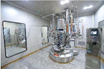
Additional Clean Room Facility, Bidar
